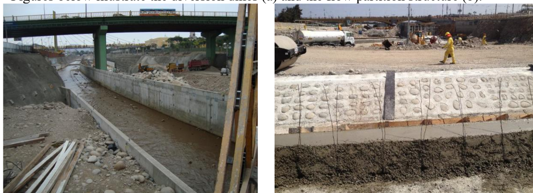
Figure 3. (a) Diversion channel constructed for the works and (b) diversion dike directing the river flow.
