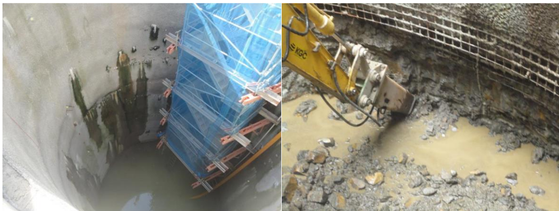
Figure 9: Detail of Shaft 2 showing (a) beginning of water drainage and (b) excavation with pick hammer in a saprolitic residual soil section. (Source: ATO GeoCompany).
