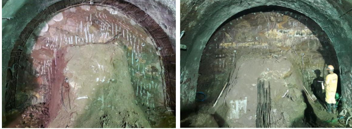
Figure 6. View of the excavation face showing (a) the CCPH columns and (b) the forepiling. (Source: GeoCompany Construction Supervision – ATO).
