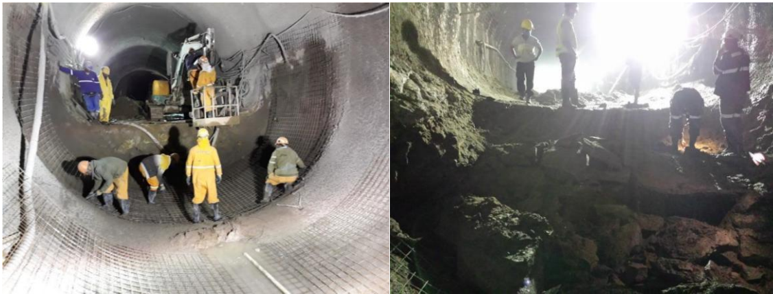
Figure 7. Reinforcement installation for final invert arch concreting and Excavation view showing the blasted rock mass. (Source: GeoCompany Executive Design).
